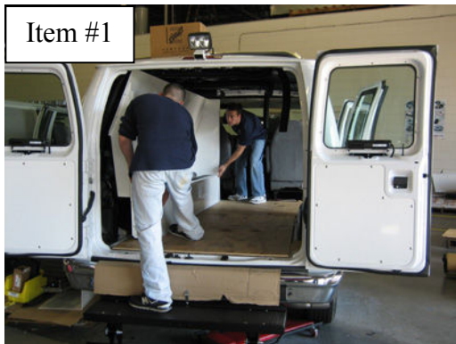
Place Driver-side Bench/Wall assembly into van so bench rests on wheel well
